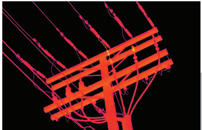
Electrical utility distribution lines
